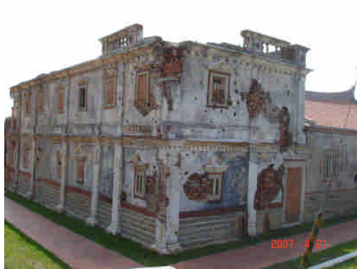
Figure3. Bullet holes on the exterior of Bei-shan Mansion.
